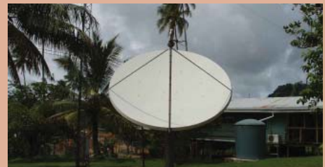
VSAT Antenna at Allied Gold's Simberi mine, PNG
