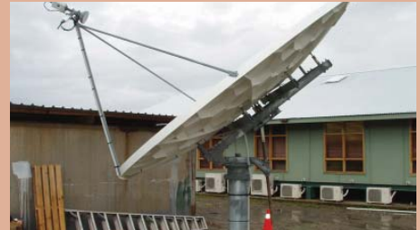
VSAT Antenna at Allied Gold's Gold Ridge mine, Solomon Islands
